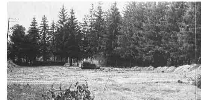
Bulldozing work begins on the future Student Center and Library Building in the area next to the former mansion.
