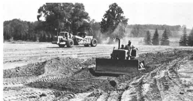
Large earth-moving equipment begins transformation of the Gierok cornfield into the Athletic Field.
