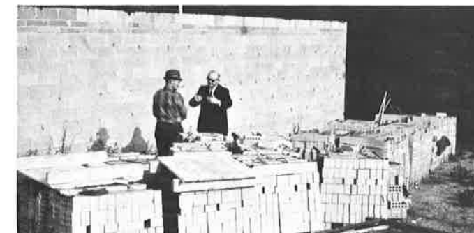
Another addition to the Multi-Purpose Building for Bookstore use attracts the attention of President Palmer.
