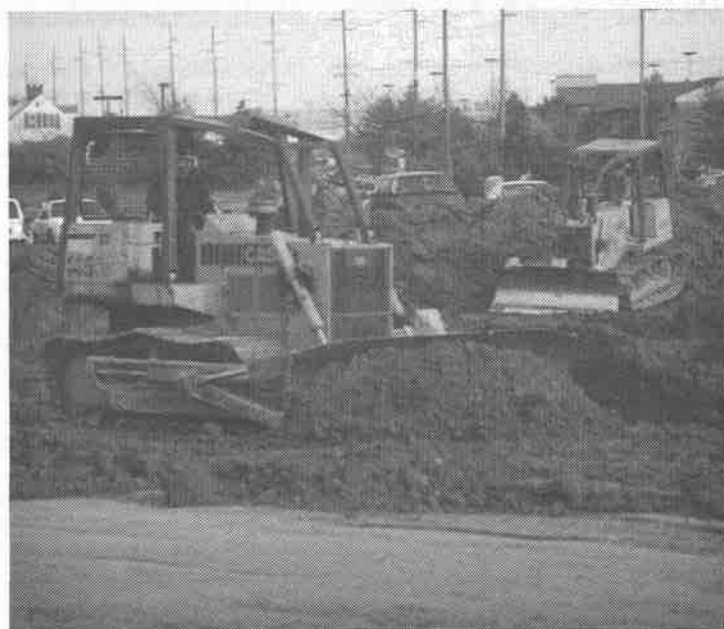
Moving mountains. Heavy equipment levels the site of the Ennis and Nancy Ham Library. Construction began in November. Photo by Brad Irwin.
