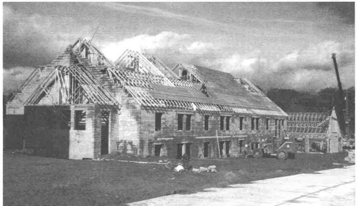
Workers install the roof superstructure on the west wing and commons area of the residence hall complex.
